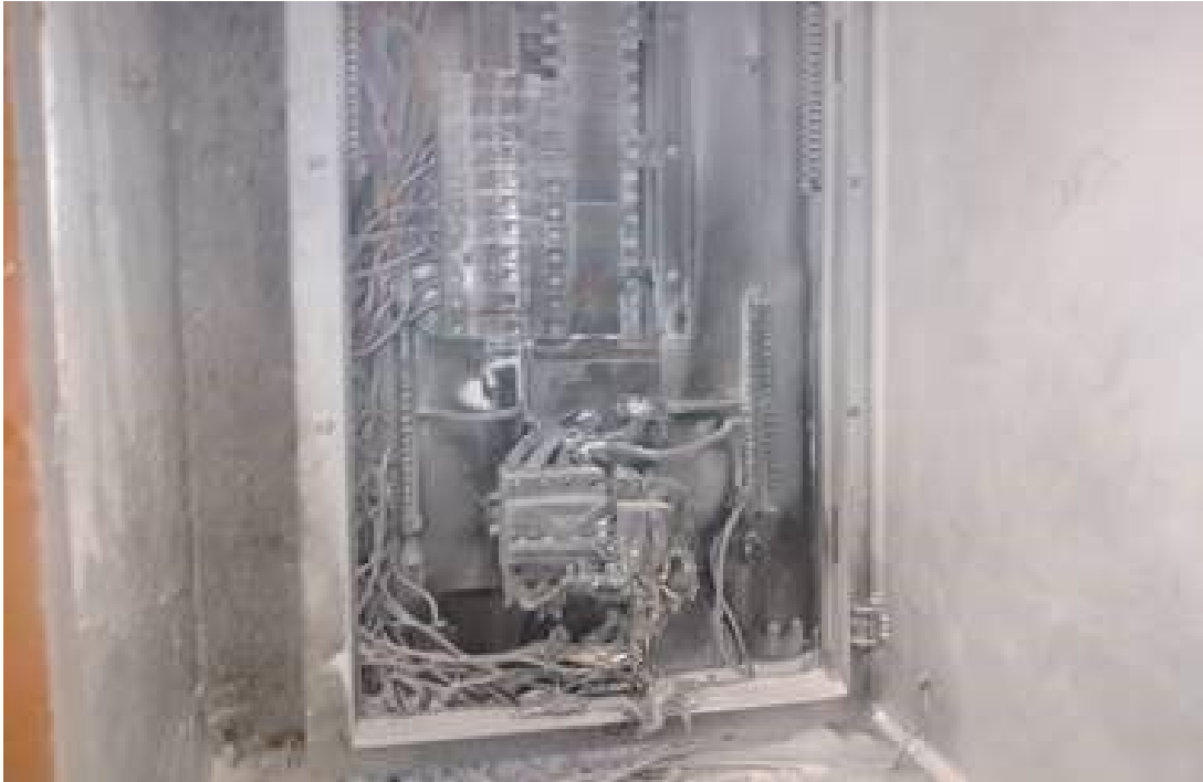
Condition of LDB after Short circuit in RCCB
